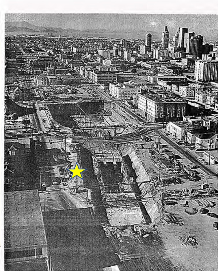
Overview of Lake Merritt Station construction showing the interface with completed subway structures, Oak Street detour, excavation and support, and extent of construction progress on the station structure. Contract 1X0071, Subway Structure, Lake Merritt Station.
